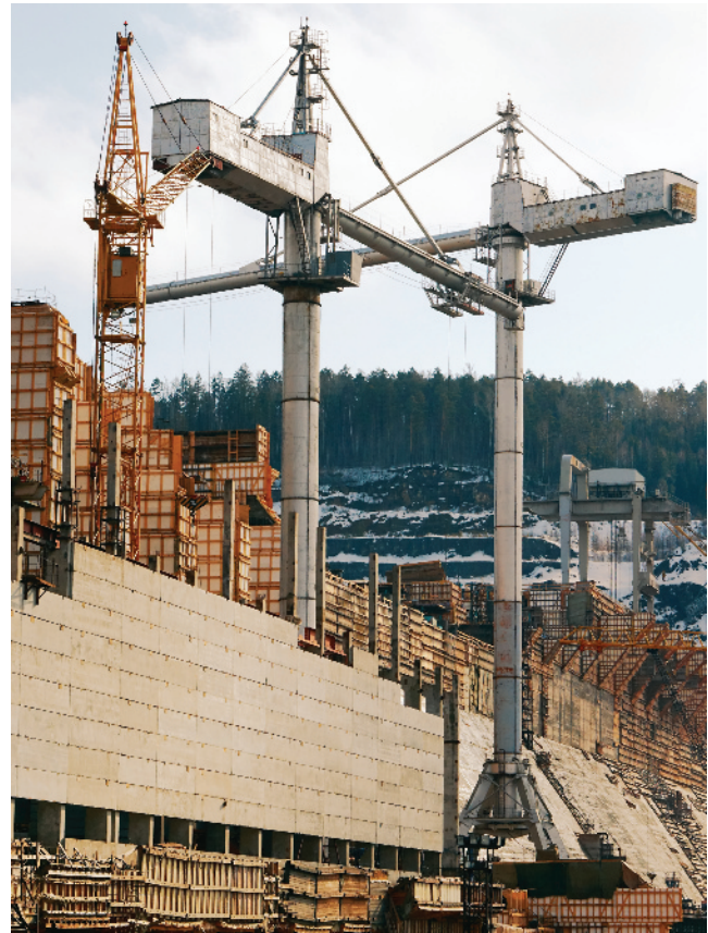
Figure 1.3 “Heavy construction” is the term used for larger infrastructure projects, such as highways, bridges, and canals.
